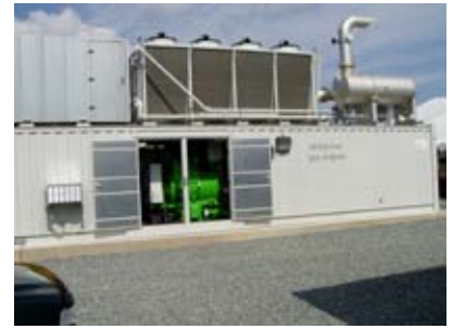
R-Board Ameresco Stafford, LLC 2.1 MW LFG
