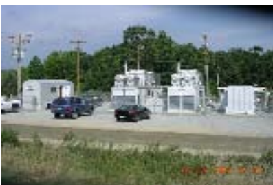
Landfill Gas to Energy
