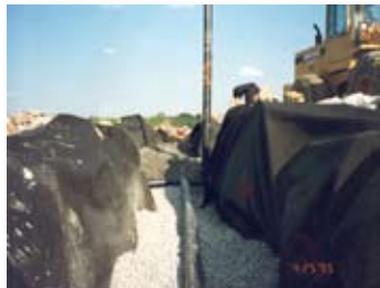
Active Gas Extraction System Fredericksburg, VA
