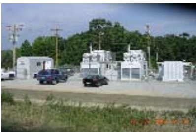
Landfill Gas to Energy
